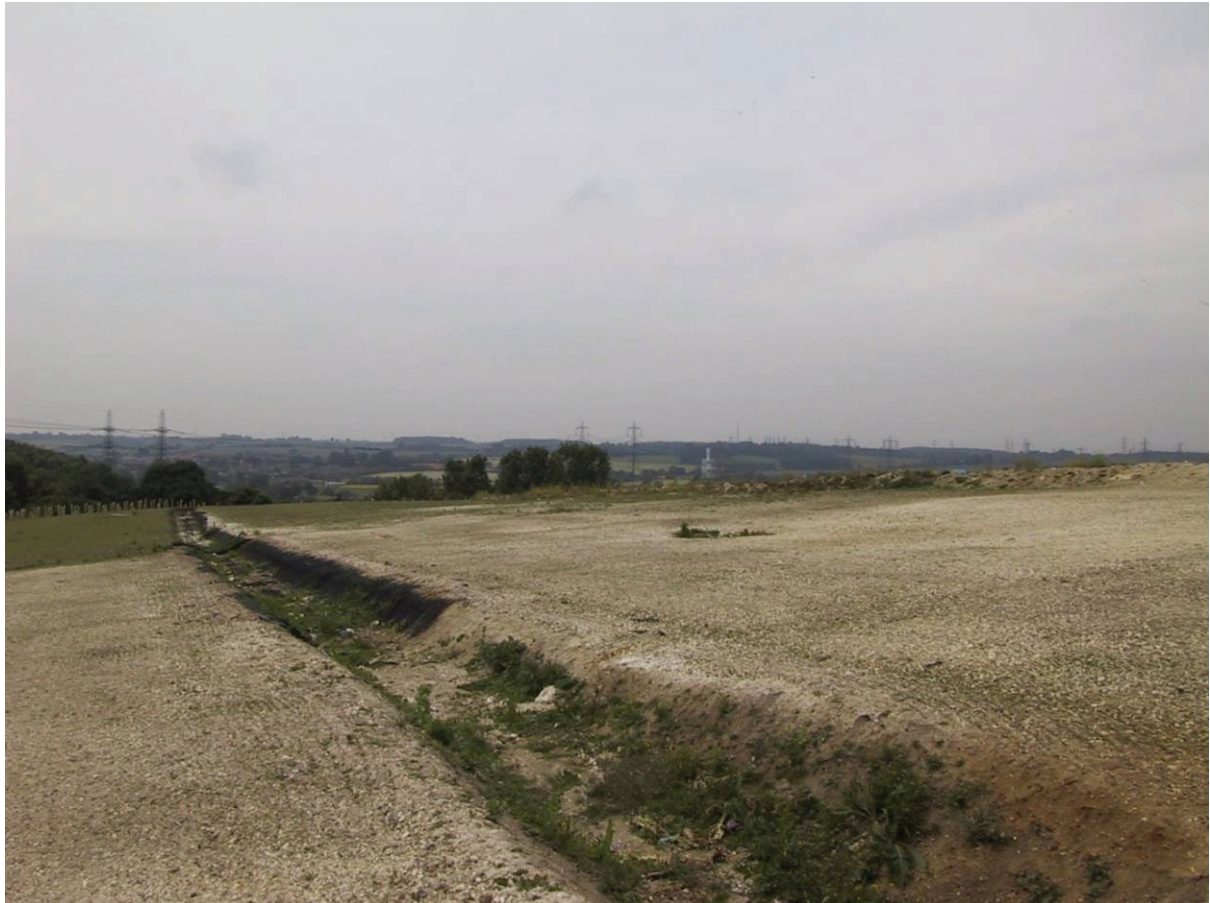
Figure 8: Bramford Landfill Site - restoration in progress. The foreground of the photo shows an area of recently established restoration substrate specifically designed to provide suitable ground conditions for the establishment of calcareous grassland. The surface water ditch at the centre of the image was lined with a permeable geotextile and then soiled and seeded for stability. In the background on the left hand side of the image a calcareous sward and deciduous woodland stand are already maturing and diversifying floristically. Photograph © SLR Consulting Ltd.
