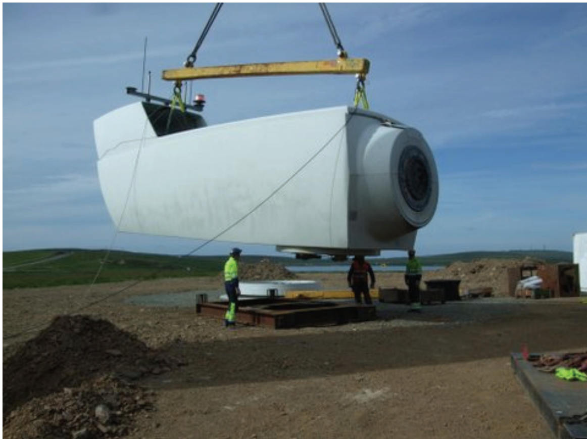
Figure 3: Lowering of wind turbine nacelle at Spurness Wind farm, Orkney. Courtesy SSE Renewables.
