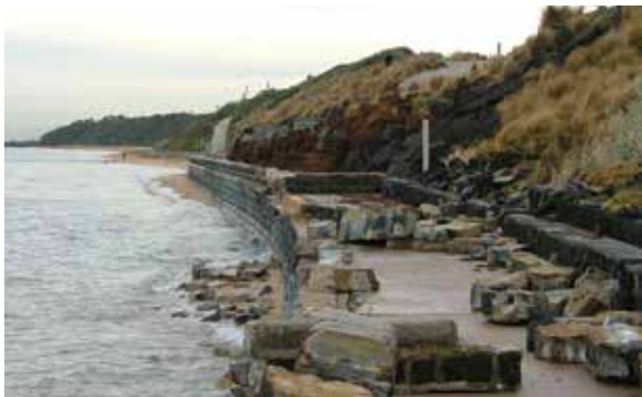
Bluestone masonry seawall at Black Rock, constructed in the 1930s, has sustained significant storm damage. A rock revetment along the existing seawall is to be built to protect the historical bluestone seawall, promenade and adjacent cliffs from erosion. Photo: M Mitchell
