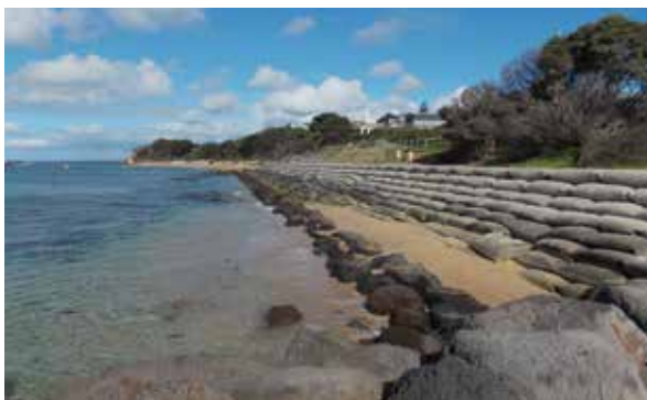
Temporary sandbag seawall at Portsea front beach, to be replaced by a rock revetment. Photo: R Molloy
