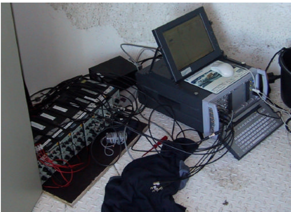
Figure 11 Measurement equipment installed in turbine tower
