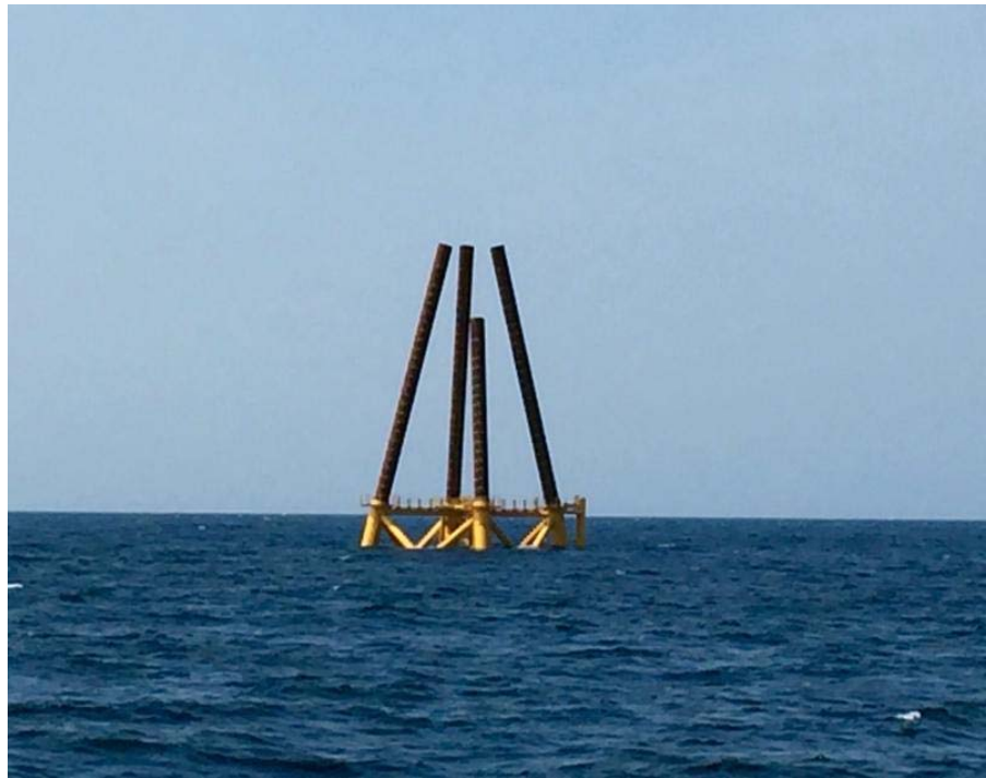
Figure 3.4. Photo of jacket foundation after piling, showing the steel piles in the jackets, through which they were piled into the seabed. Source: Block Island offshore wind farm, US.
