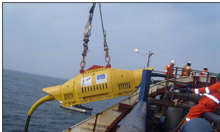
Figure 3-45: Cable Connector Lowered into Place from Cable-lay Ship at Wave Hub, August 2010 (JDR Cables)
