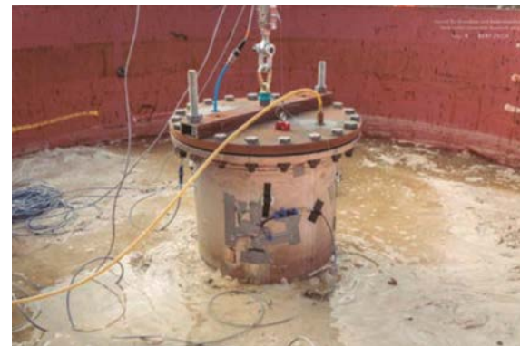
Fig. 1 Decommissioning with overpressure – sealed pile head equipped with pressure and strain sensors
