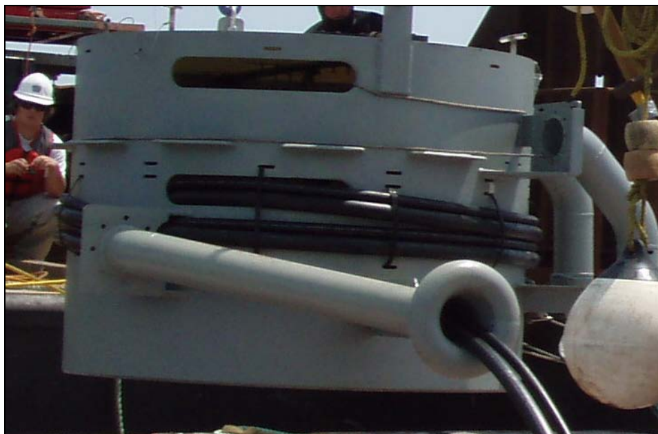
Figure 14. Shore cable termination anchor
