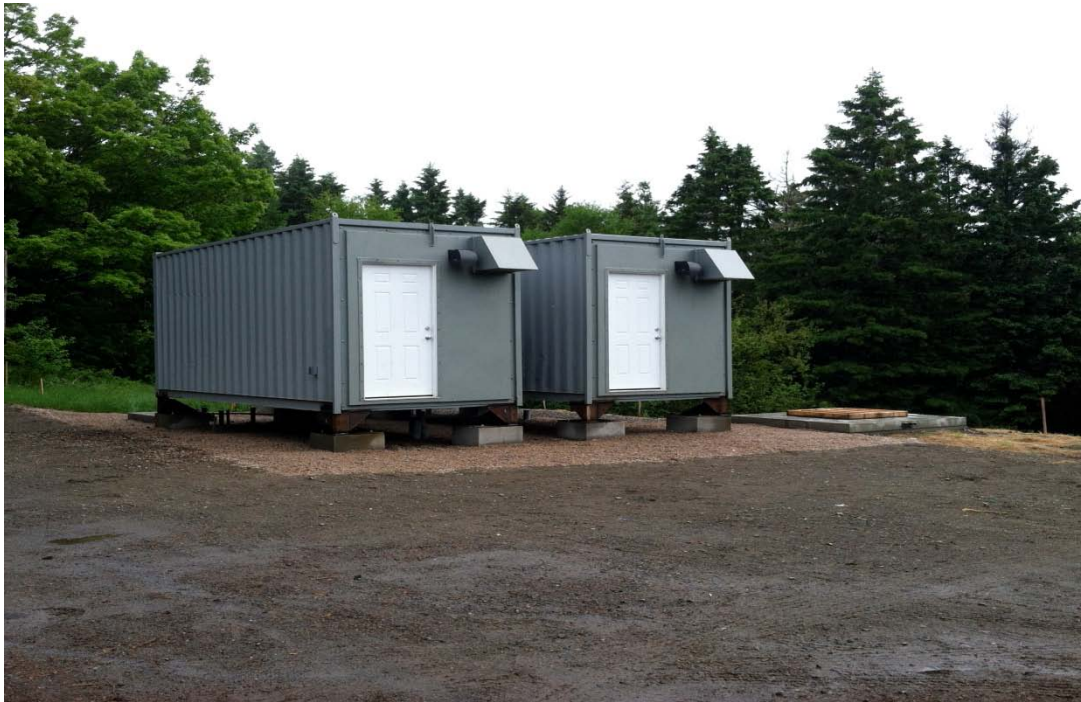
Figure 20. On-shore Station, Lubec, Maine.
