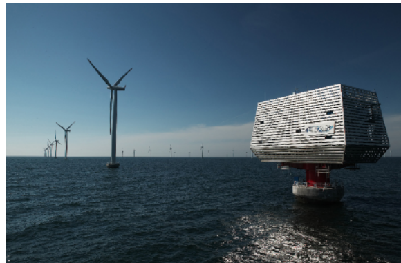
Figure 3.4 Offshore substation at Nysted Offshore Wind Farm (Denmark)
