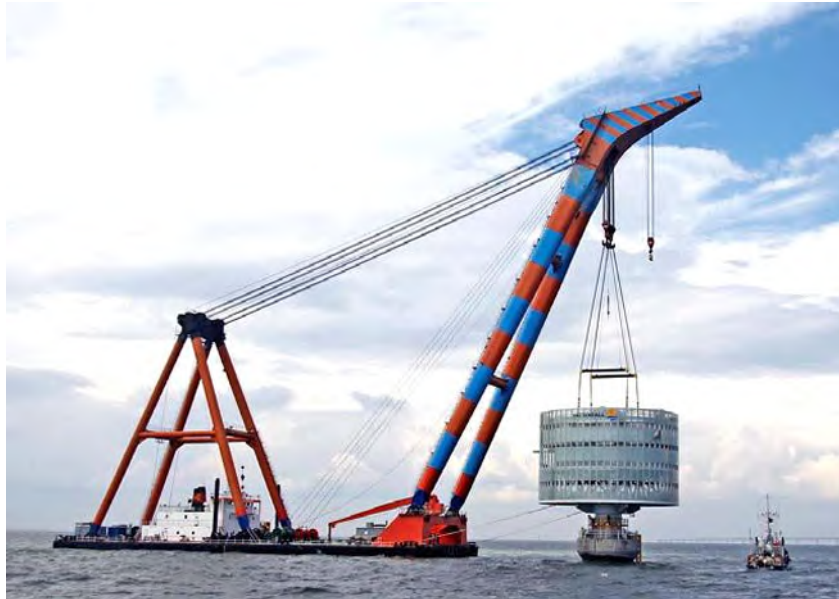
Fig. 1.2.4. Installation of power substation in the Lillgrund wind farm (photo by Jeppsson et al. 2008).
