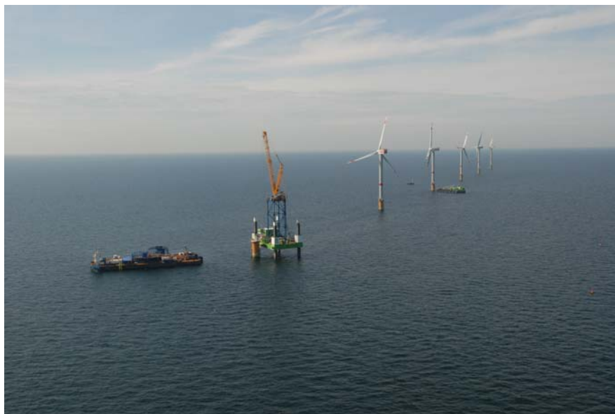
Figure 3. Image of the activity at the Thorntonbank windfarm site on 9 September 2008, showing the cable barge which was also present on 10 September, when underwater noise measurements were made (photo MUMM / RBINS).
