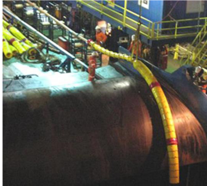
Figure 5.15 - Example of a cable laying operation (cables first end being over-boarded from the cable laying vessel)
