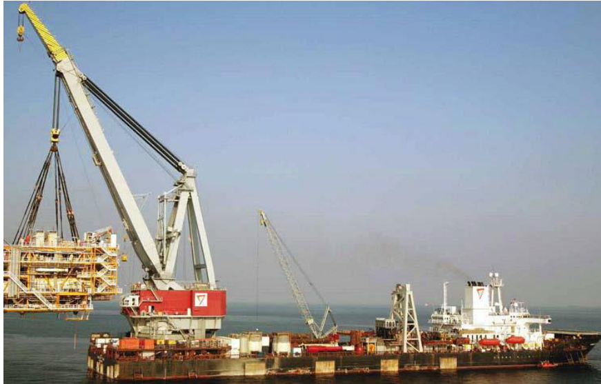
Figure 5.28 – SHL vessel performing heavy lift of a conventional offshore substation platform topside
