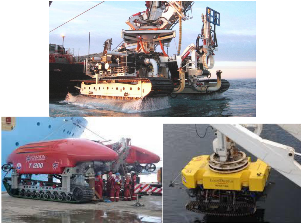
Figure 5.19 – Examples of seabed water jetting cable trenching tools and cable plough that may be used for inter-array cable installation
