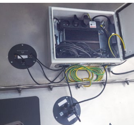
Acoustic bat recording in the nacelle: the recording unit is housed in a secure box. The two black discs indicate the position of the microphone (with test signal generator and heating, below) and the antenna for remote controlling and access (left).
