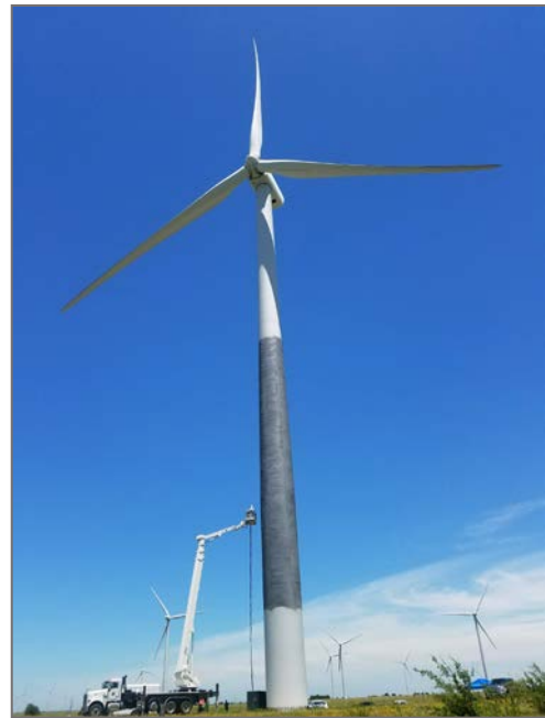
Figure 12: Texture coating application to a wind turbine tower at Wolf Ridge Wind, LLC in 2017.
