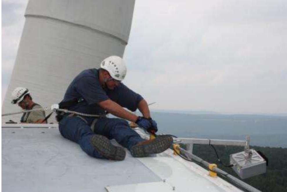
Tom McRoberts with Deaton Engineering attaches an acoustic deterrent device to a wind turbine.
