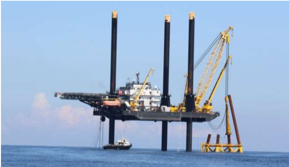
Figure 3. BIWF Phase 1 Construction Pile Driving. Top panel: Piles inserted in jacket prior to start of pile driving. Lower panel: Pile driving in progress.
