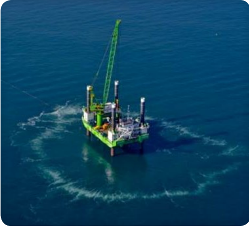
Large bubble screen - Noise mitigation during the construction work of offshore wind farm Borkum West II
