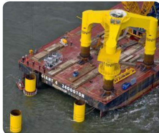
Tripile foundation used by BARD GmbH for its offshore wind parks (BARD Engineering GmbH)
